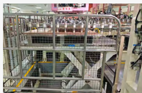
Kunshan Site Wire Mesh Installed on Machine Guards
