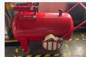
Huangshi Site Added Mobile Foam Extinguisher
