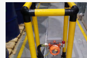
Huangshi Site Combustible Gas Detectors Added to the Chemical Warehouse
