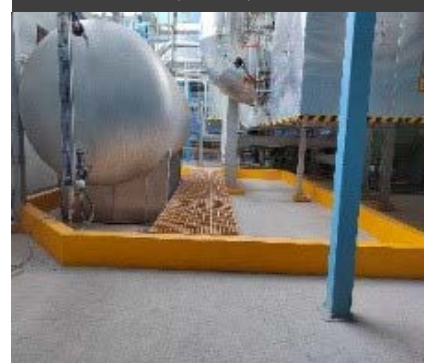
RTO熱媒油低位槽設置防洩漏圍堰
