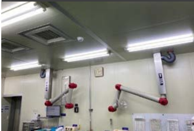
Movable aspirators were added to IQC/IPQC
